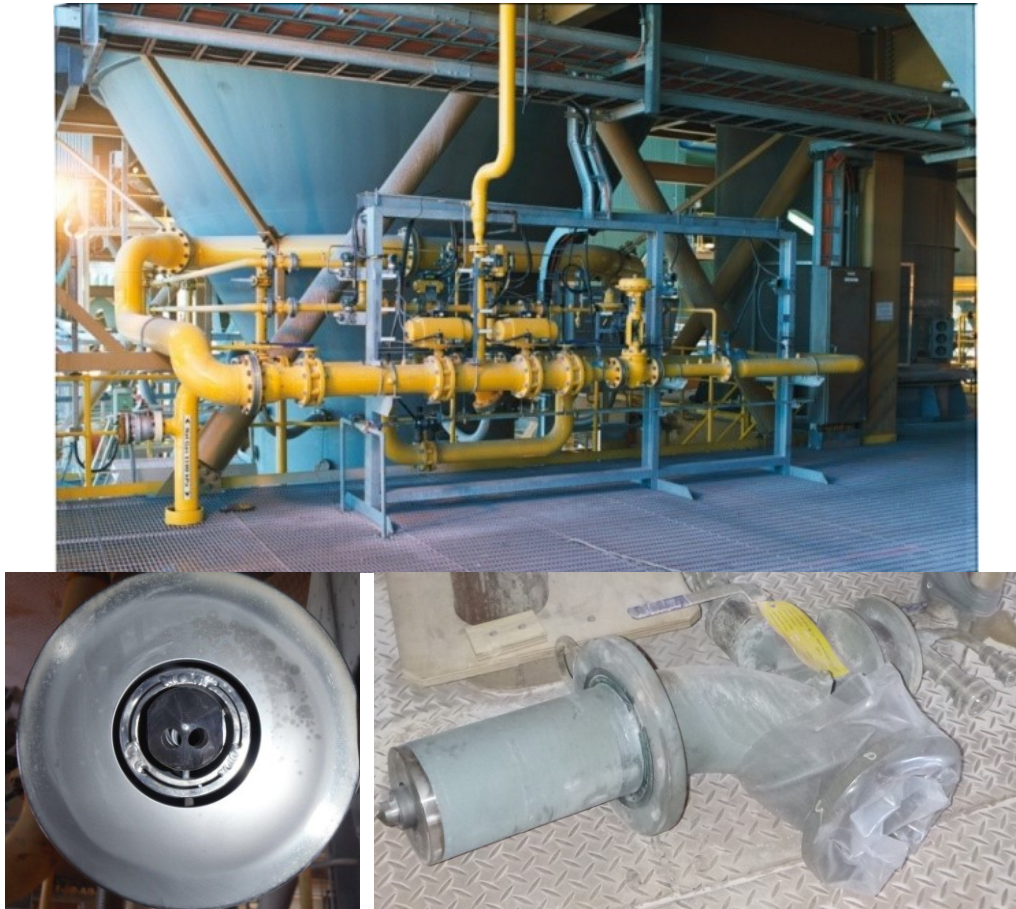
Figure 6. Picture of dual fuel burner in calciner vessel.
